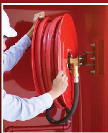
Hose Reel Pressured System
