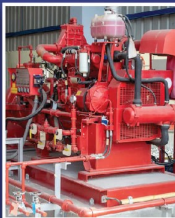
Automatic & Manual Fire Fighting Pump & Diesel Engine
