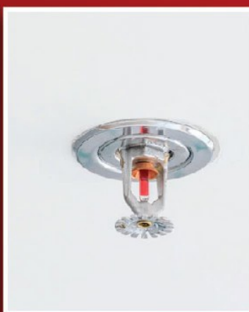
Automatic Sprinkler System & Equipment
