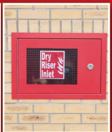
Wet & Dry Riser System
